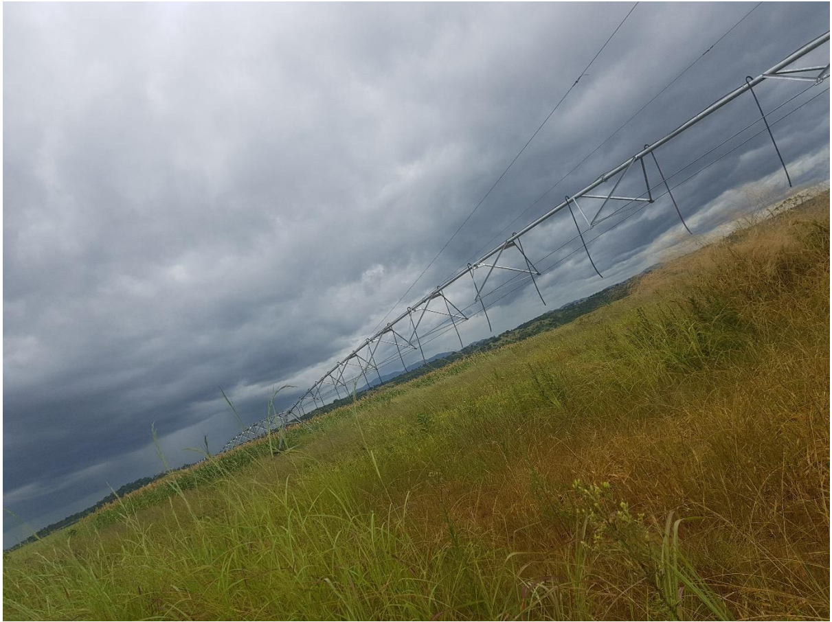
One of the four installed centre pivots
